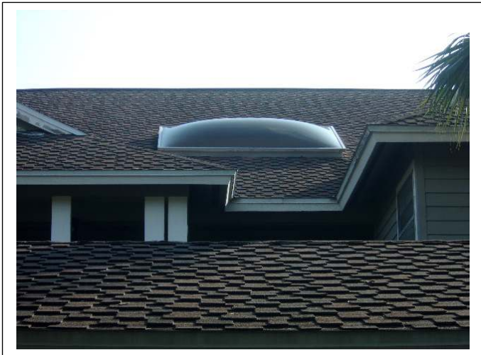
OPENING PROTECTION – The skylights are not rated or protected
