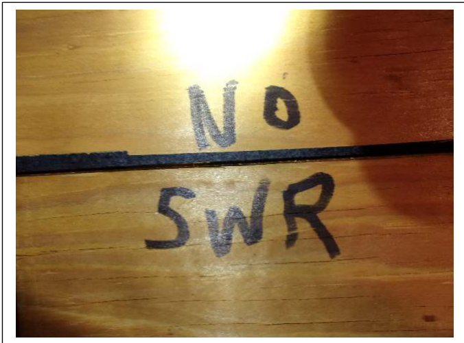
SECONDARY WATER BARRIER – Is not installed
